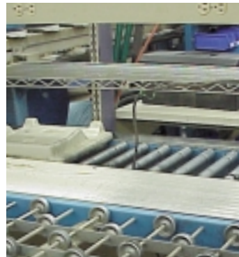
Hytrol skatewheel and powered roller conveyors in progressive mechanical assembly.
